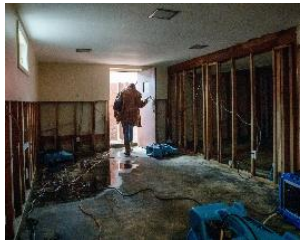
Sewer flooding: inside your property
